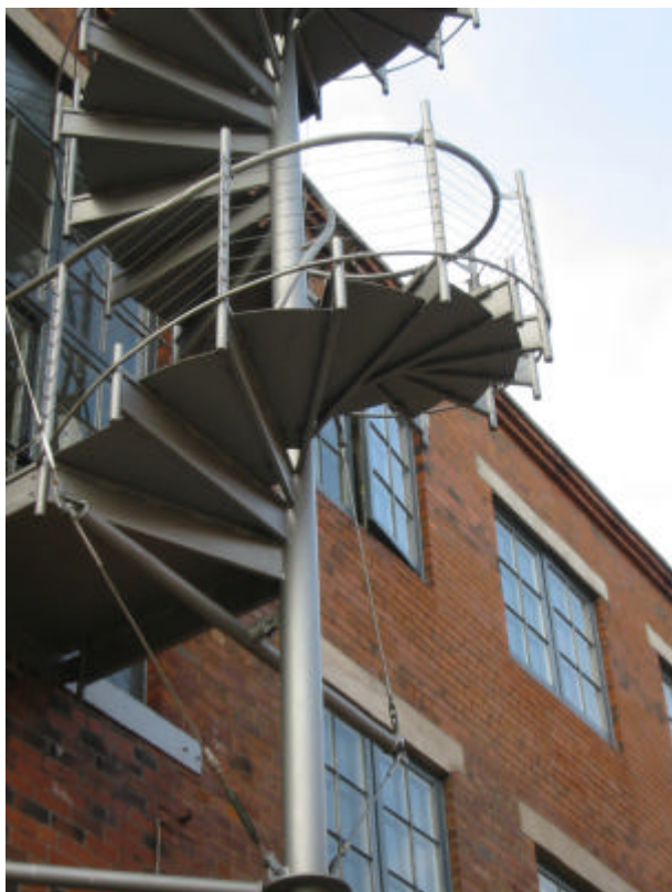
The use of steel as a construction material can create interesting design features and reflect the area's industrial past
