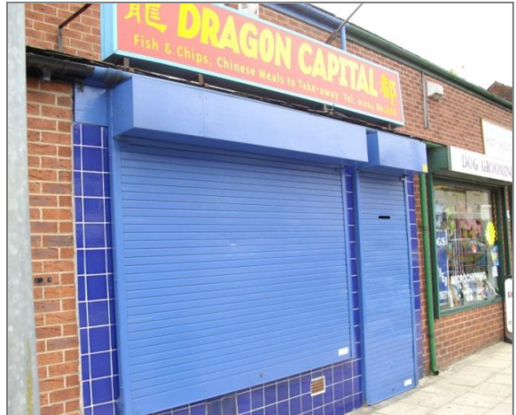
Solid Security Shutters with protruding external shutter boxes are not acceptable
